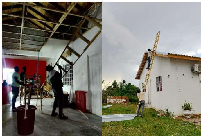
Restoration work underway at the Y's Menettes Resource Centre in Savanna-la-Mar during May 2026.
